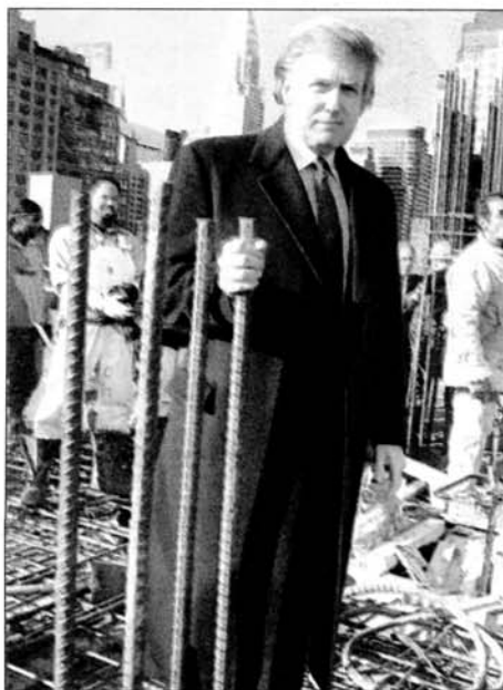
The most prominent developer of all, Donald Trump (shown during construction of the Trump World Tower) advises wannabees they'd better: "Be prepared not to like sleeping."
