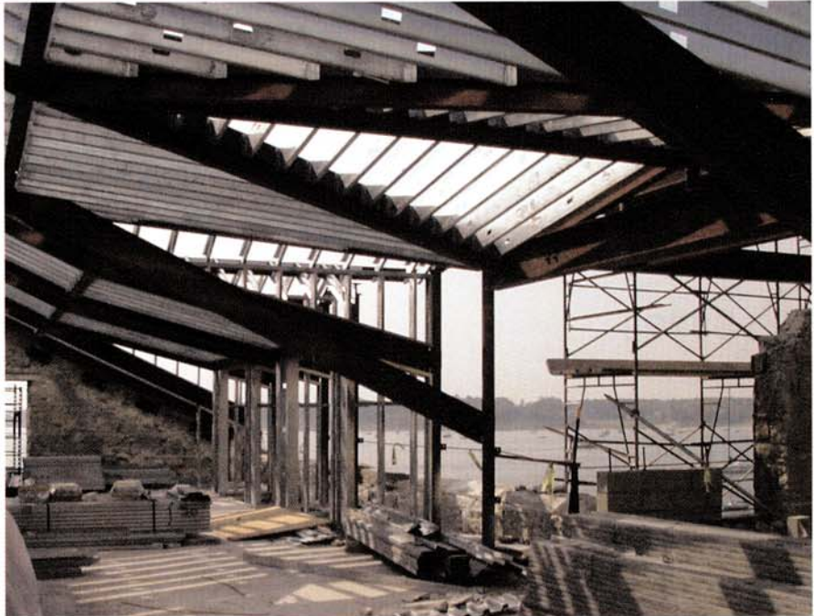
View from the historic 1849 Trumbull Building looking out from the upper floor into Stonington Harbor. A fire required major rehabilitation of the granite structure.
